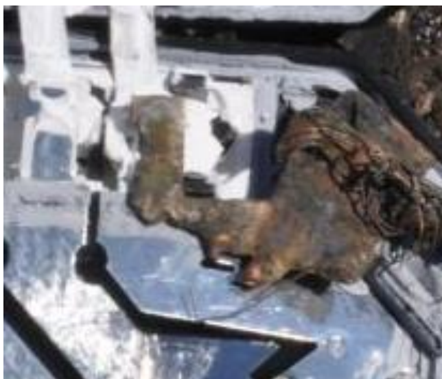
Figure 14: Damaged part of a PV module junction box laid over an identical undamaged component, showing where material has been ablated through arcing.
