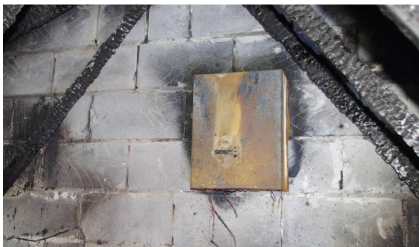
Figure 13: Inverter fire with clear burn patterns showing this as the source of the fire.
