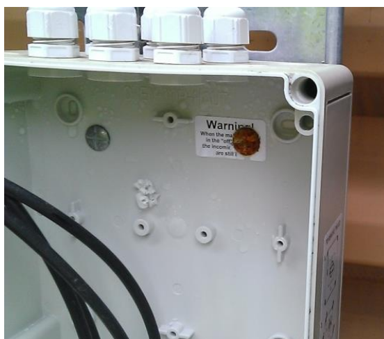
Figure 9: Rear of isolator enclosure drilled through for mounting screws. Note that the screw on the right hand side is rusty, indicating water ingress.
