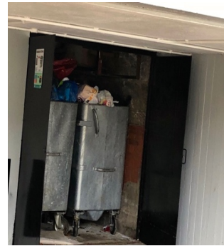
Refuse storage at the bottom of chute
