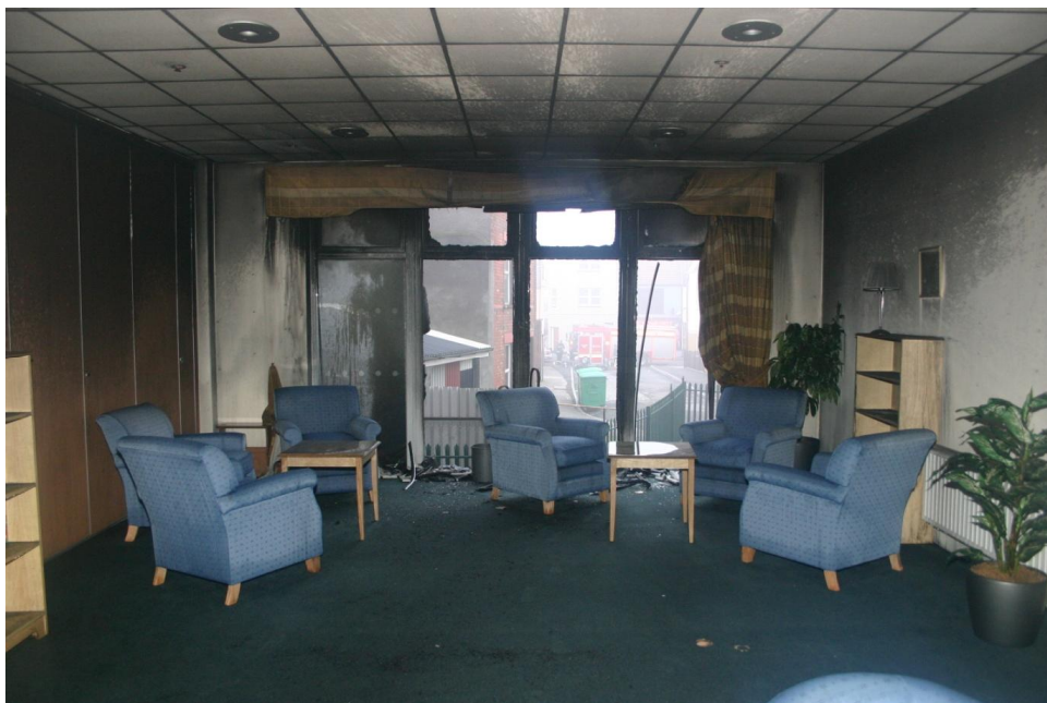
Figure 13 - Fire spread from broken windows controlled by sprinklers (Photograph courtesy of Avon Fire and Rescue Service)
