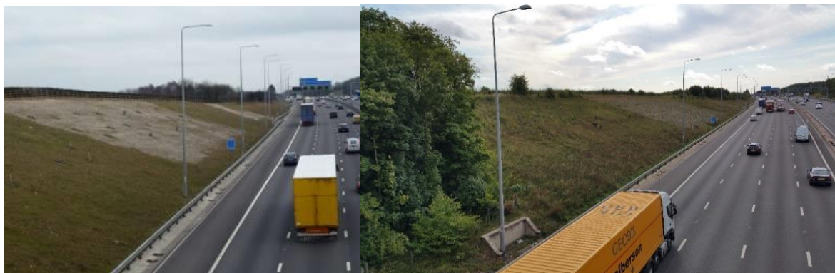
Figure 5-5 Areas of poor establishment of grass seeding near Selston recorded at OYA (left), showing signs of establishment at FYA (right)
