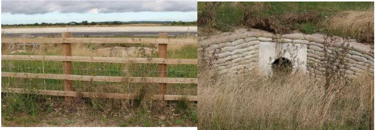
Figure 5.11 (left) illustrates HB fencing with mammal tunnel entrance within highway verge area. Figure 5.12 (right) is close up of the mammal tunnel entrance WU4.
