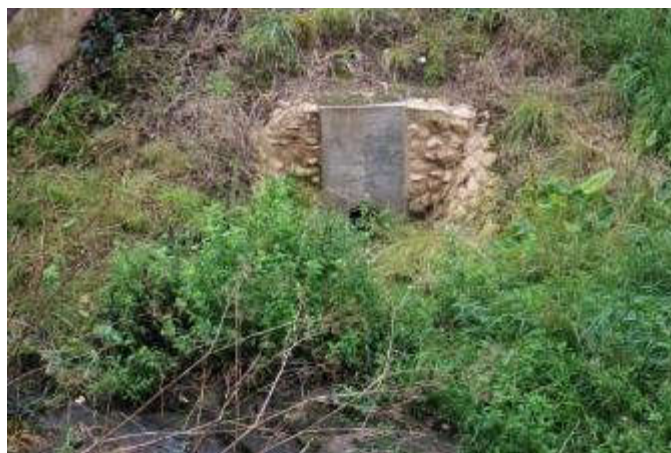
Figure 5.27 Example of culvert outfall at Nethergate stream which would benefit from clearance
