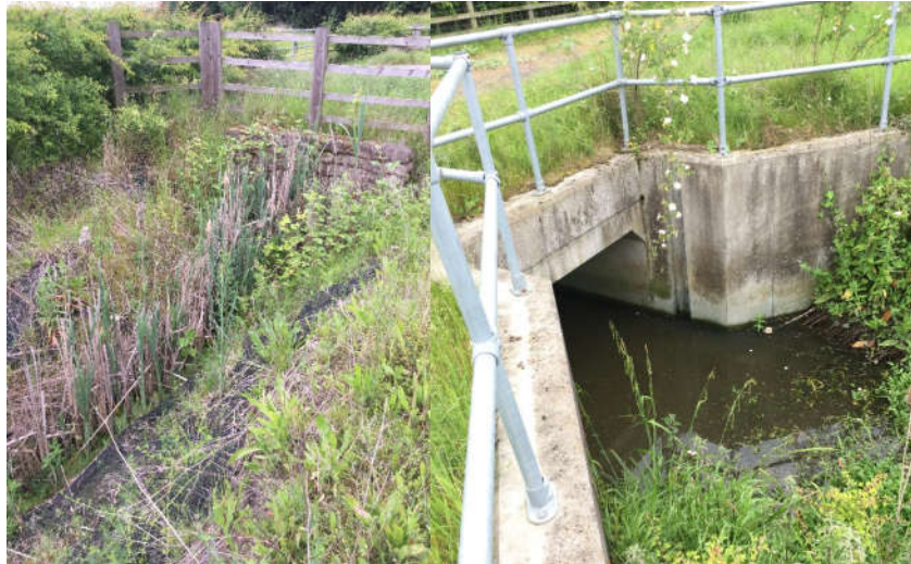
Figure 5-21 Drainage channels not receiving proper maintenance
