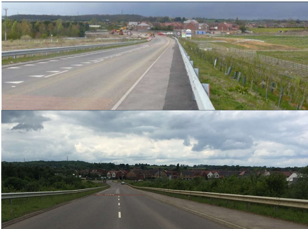
Figure 5-1 Development east of Fields Road overbridge – under construction (OYA view) and nearing completion (FYA view)
