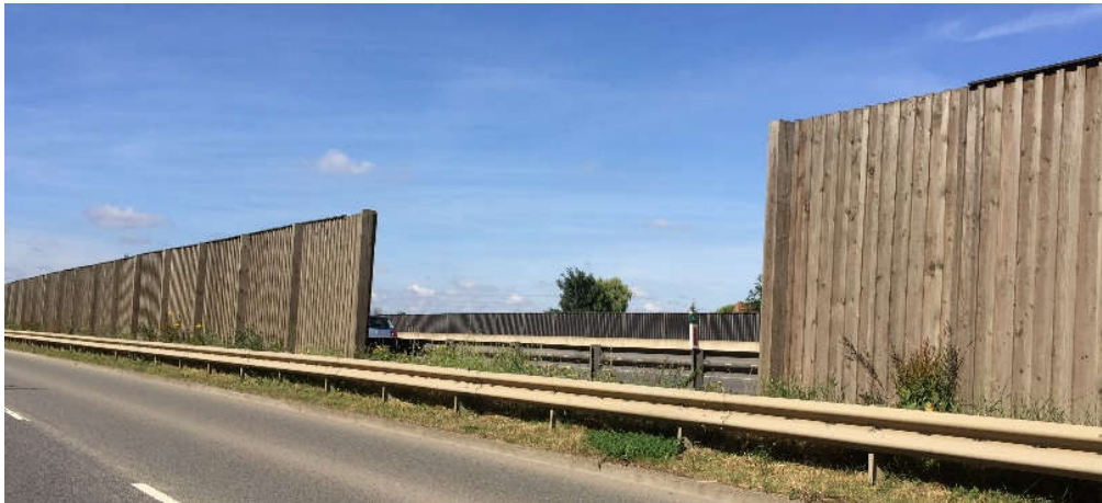
Figure 5-3 Gap in noise barrier east of Marston junction
