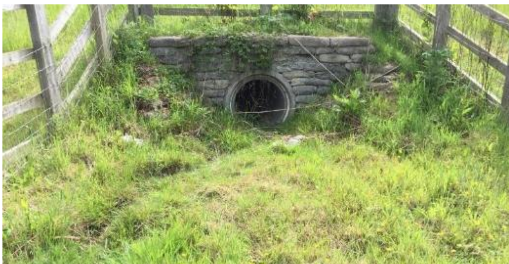
Figure 5-12 Mammal Tunnel BT02
