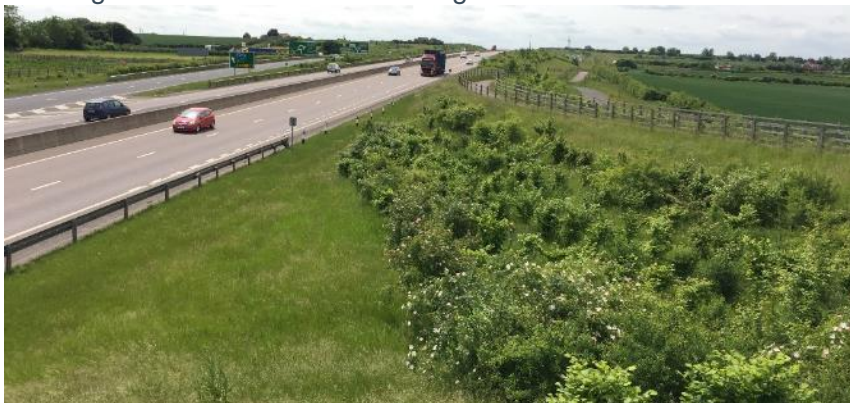
Planting north east of Hawton Lane overbridge – minimal growth with suspected compaction as an issue
