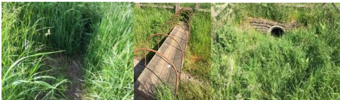
Figure 5-15 Mammal Tunnel BT11
