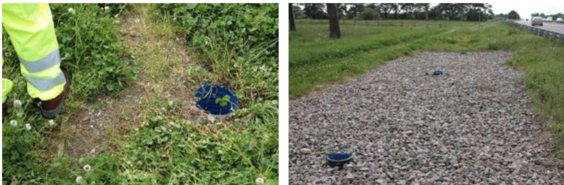
Figure 5-16 Missing Drainage System Cover
