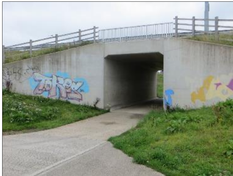
Figure 5-3 Footpath Condition and Graffiti at Sherbourne Roundabout
