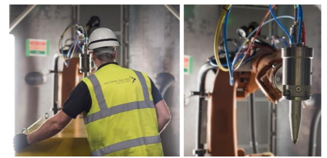
Photographs of the Laser Cutting Rig for Size Reduction of Glove Boxes at NNL Workington. Images Courtesy of NNL.
