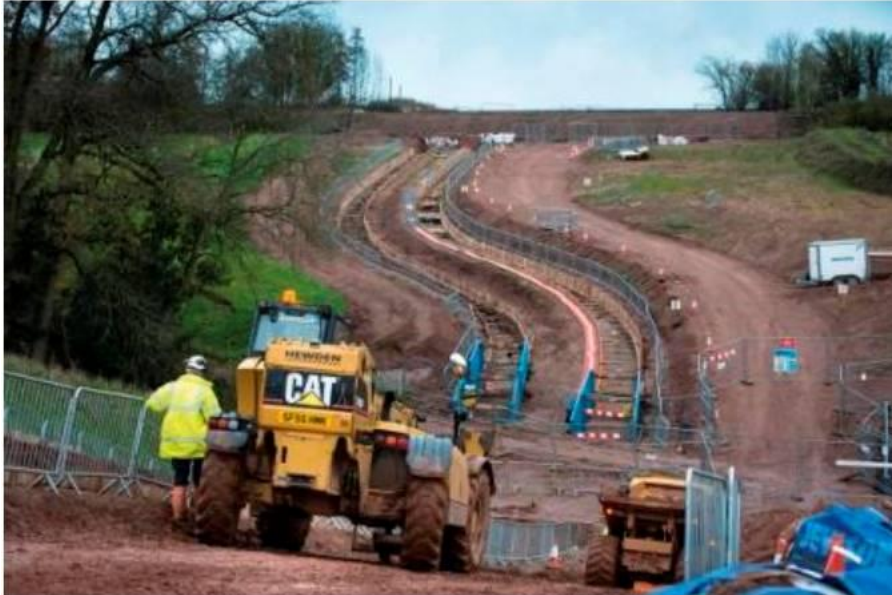
Figure 8 Visual illustration of the typical scale of working area and disruption of a two circuit cabled alignment (AP2 GSP is a 3 circuit cabled alignment)
