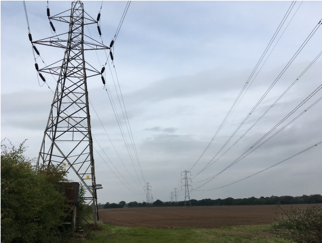
Figure 3: An indicative example of two parallel lines of pylons
