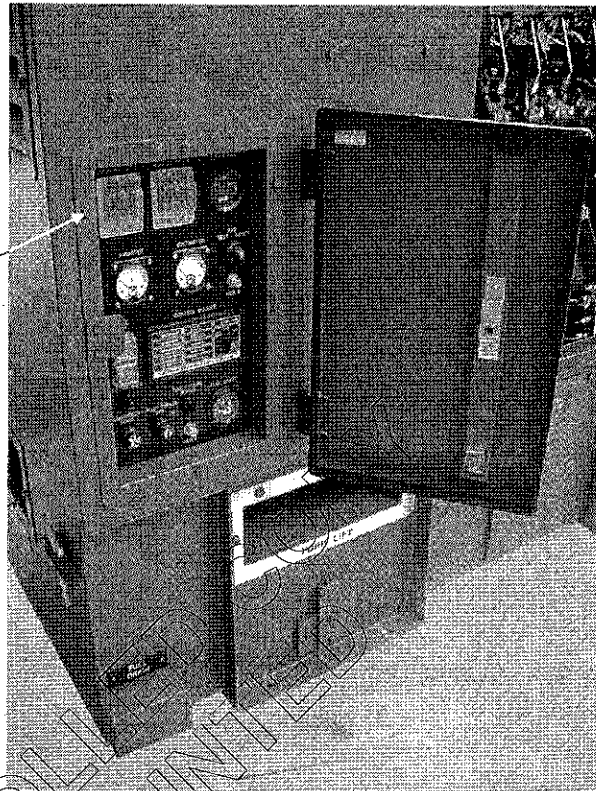
Fig 3 Control panel and door
