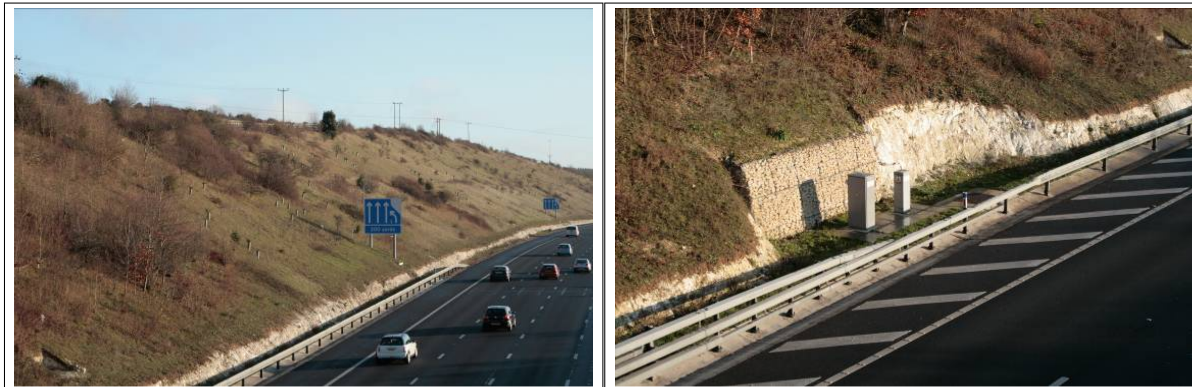
Figure B.4 – POPE views looking east from Hill Road overbridge: Views illustrates new signage, relocated cabinets, open chalk verges (as before) and retained/reinforced vegetation on cutting slopes
