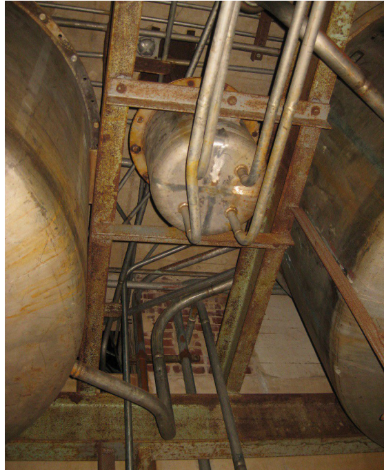
Complex networks of pipes and vessels present a significant decontamination challenge at Sellafield
