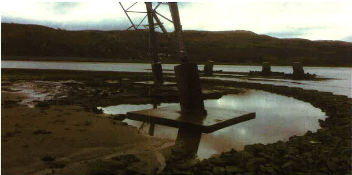
Photo 2. Loss of fine sand within cofferdam due to scour and washout
