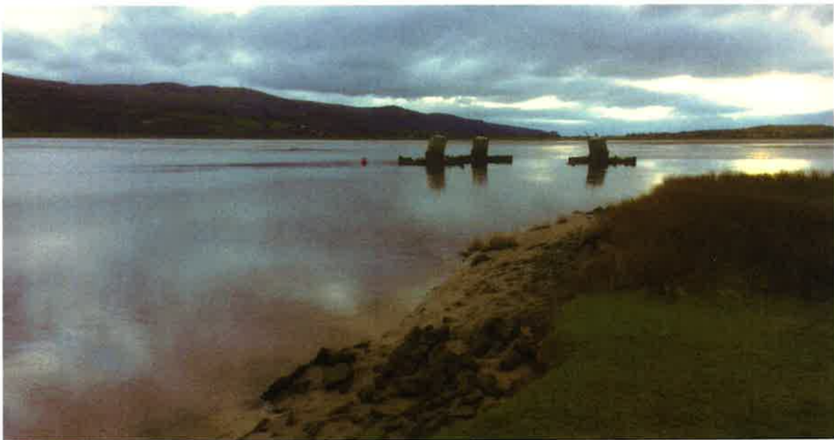
Photo 4. Ongoing erosion to the east of the cofferdam
