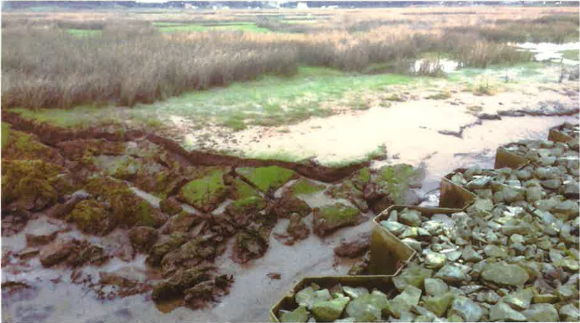
Photo 3. Ongoing erosion to the west of the cofferdam
