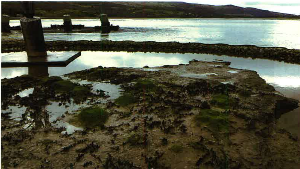
Figure 5. Scour around south leg of 4ZC030T looking southeast
