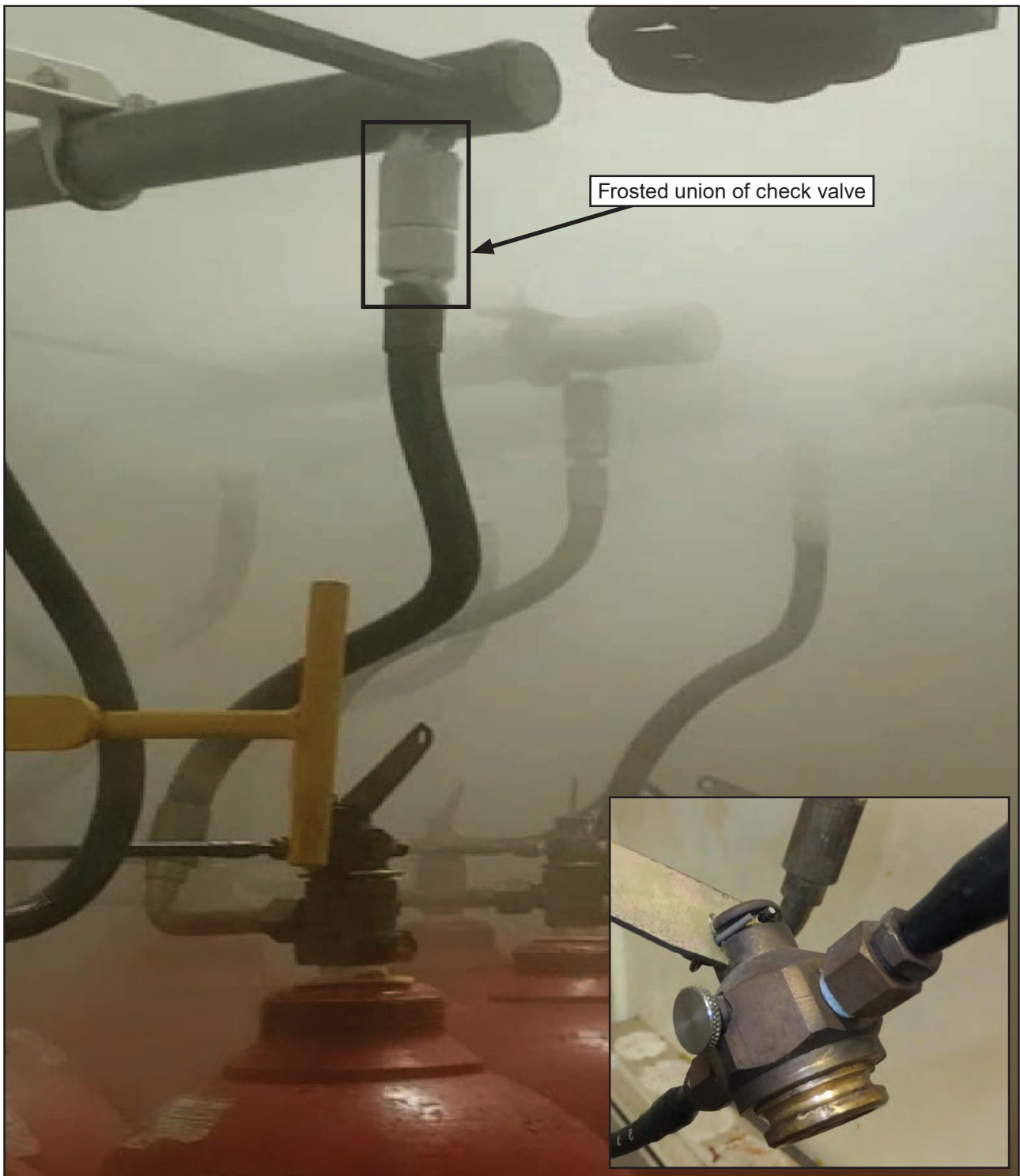
Figure 8: Dense white cloud in CO 2 room (inset: cylinder valve actuation head)
