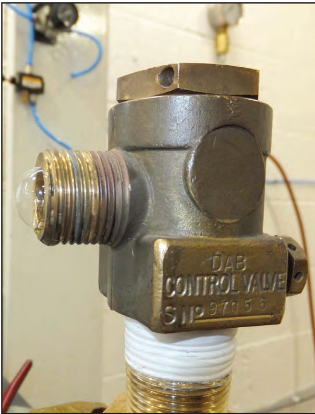
Figure 12a: Leaking DAB valve 97056
