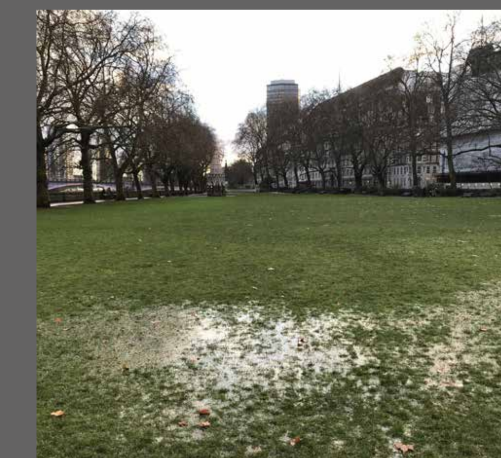
Grass to be re-laid to limit waterlogging. Image courtesy of Gustafson Porter + Bowman
