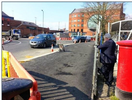
Narrow path outside rail station, widened and converted to a shared cycleway (after).
