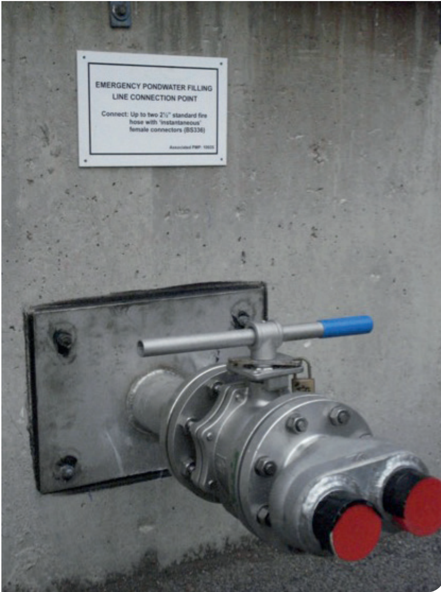
Figure 11: Emergency Pond Water Filling Line at Oldbury
