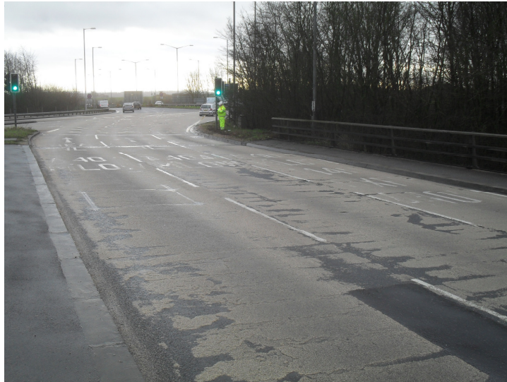
Figure 4.1 – Poor condition of existing anti-skid surfacing and road markings (view looking south)
