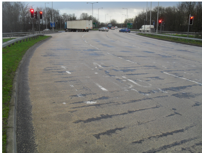
Figure 4.4 – Very poor condition of road markings on circulatory carriageway
