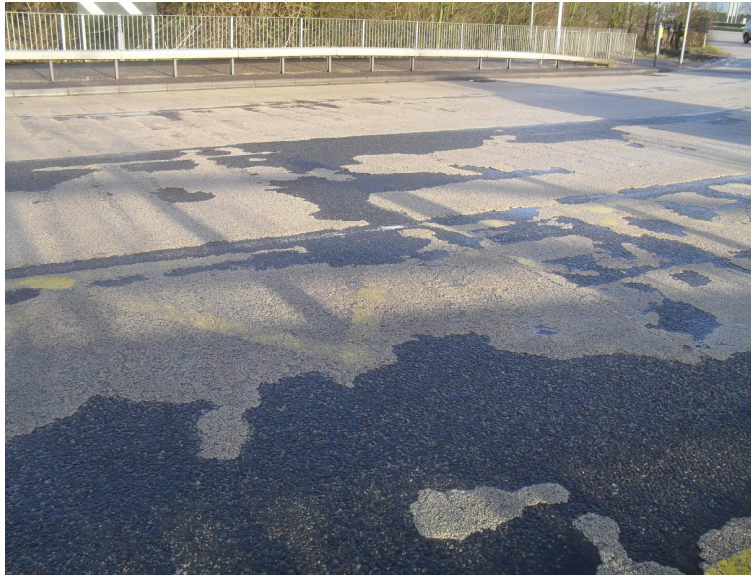
Figure 4.3 – Delamination of anti skid surfacing on circulatory carriageway
