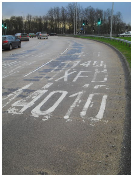
Figure 4.5 – ‘Wear’ of anti skid revealing previously applied road markings
