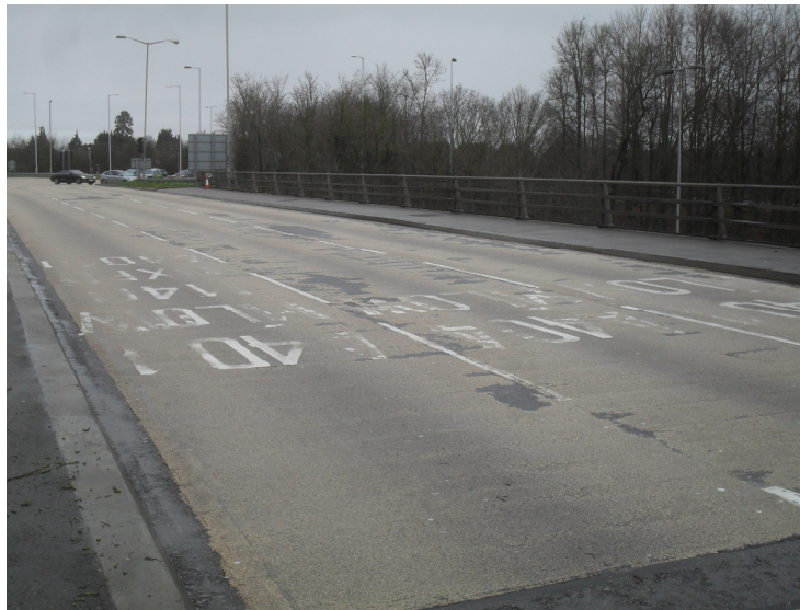
Figure 4.2 - Poor condition of existing anti-skid surfacing and road markings (view looking north)
