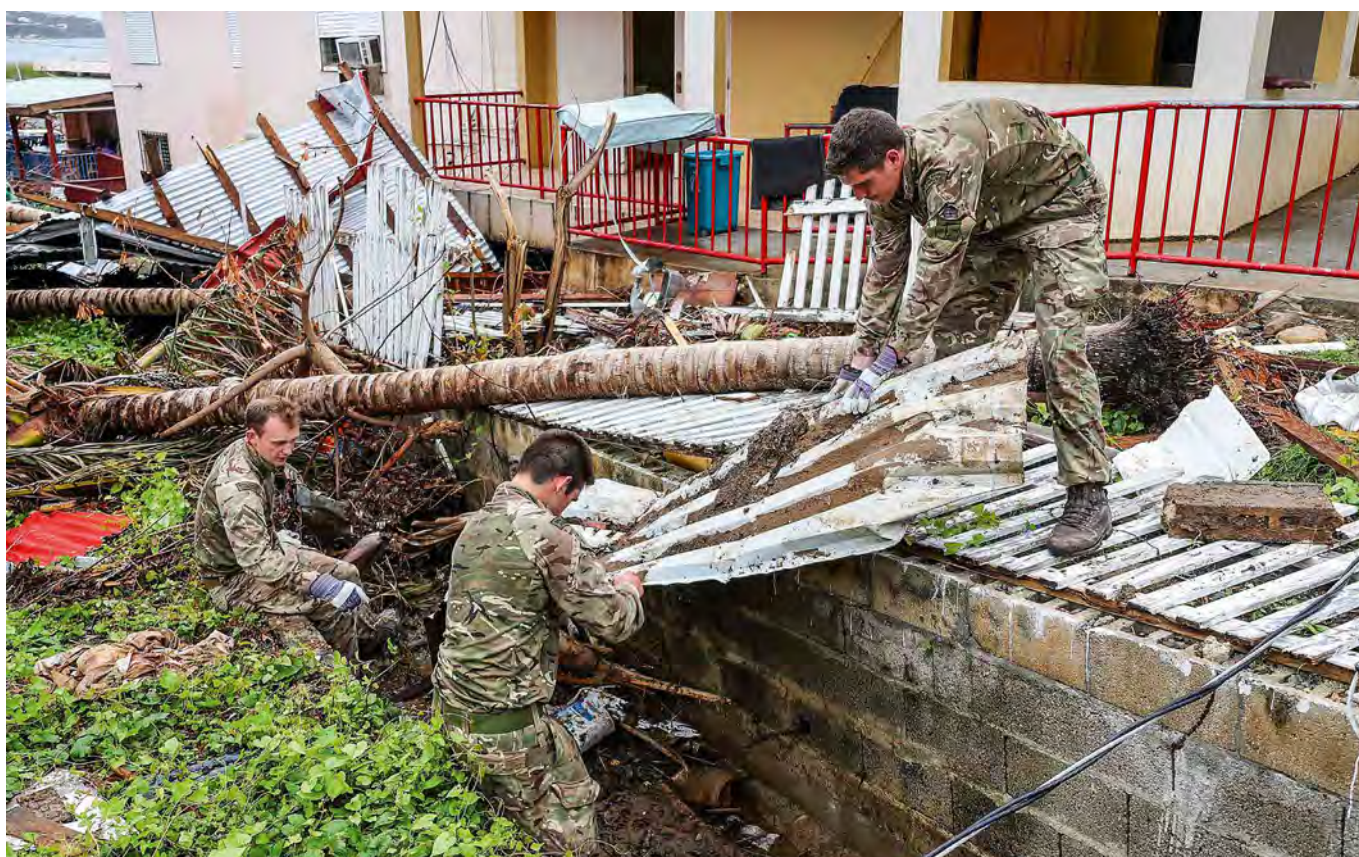
Assault Engineers from 40 Commando and Royal Engineers from 54 Commando Squadron cleared storm drains in key locations before hurricane Maria made landfall on the British Virgin Islands later that day
