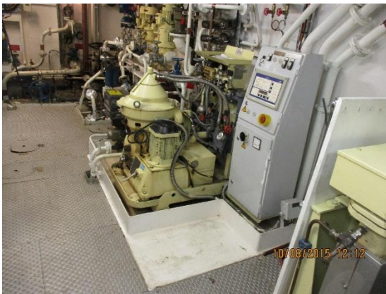
Purifier area – kept clean despite the challenge of such a space
