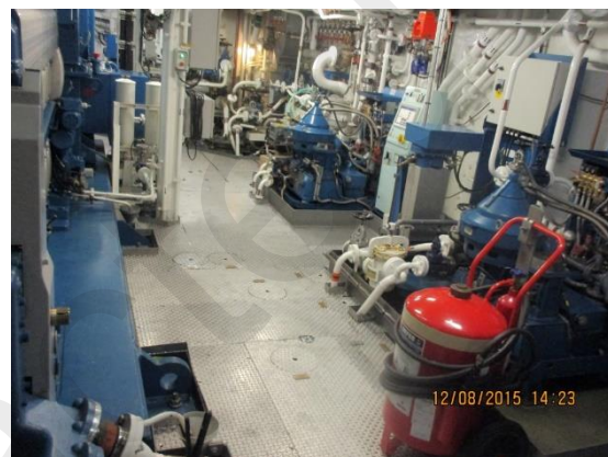
Purifier space in the main engine room - well maintained and very clean
