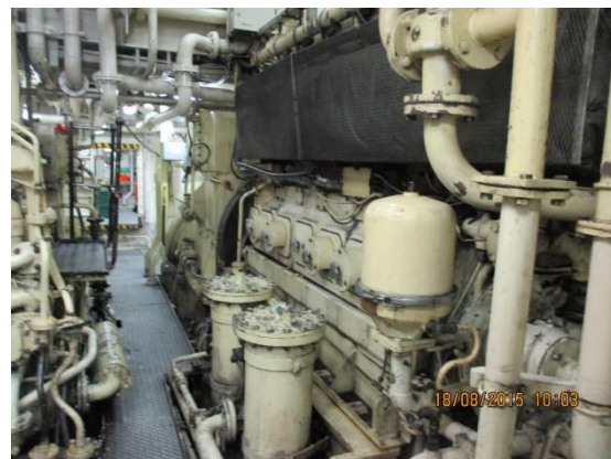
One of the Ruston 6RKcZ 750kW Engines
