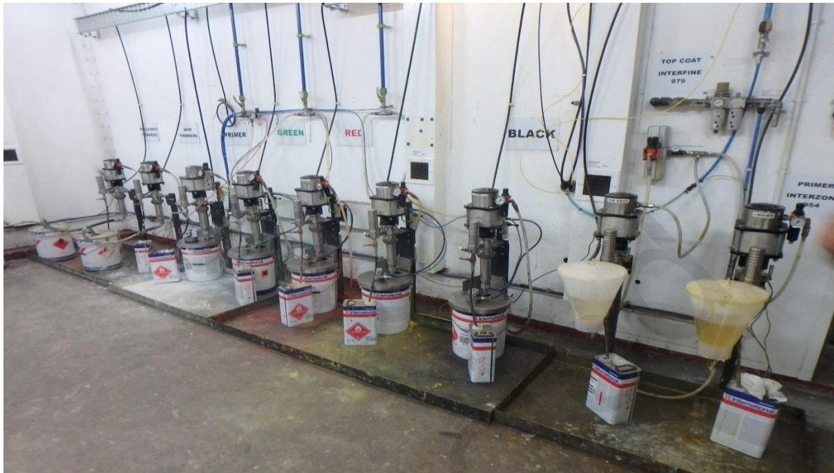
Photo 35 Paint mixing system.
