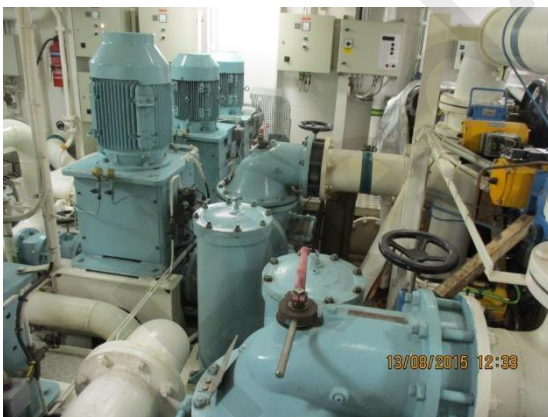
Sea Water Pump area on the Engine Room lower level. All clean and well painted
