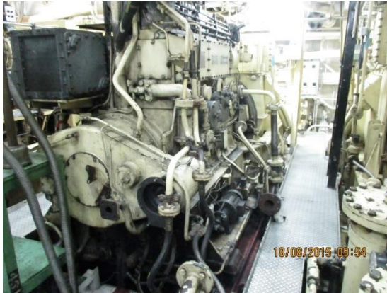
Forward smaller unit with parts missing.
