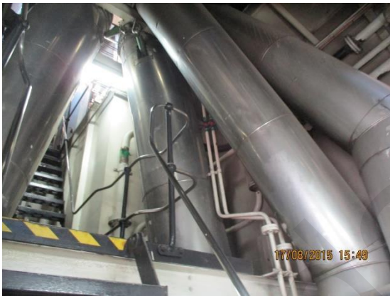
Main Engine uptakes in exceptional condition and very clean
