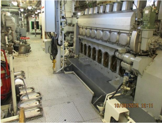
One of the 5 Wartsila Main Generator Units
