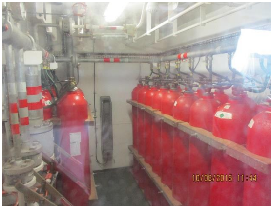
Engine room protected by CO 2
