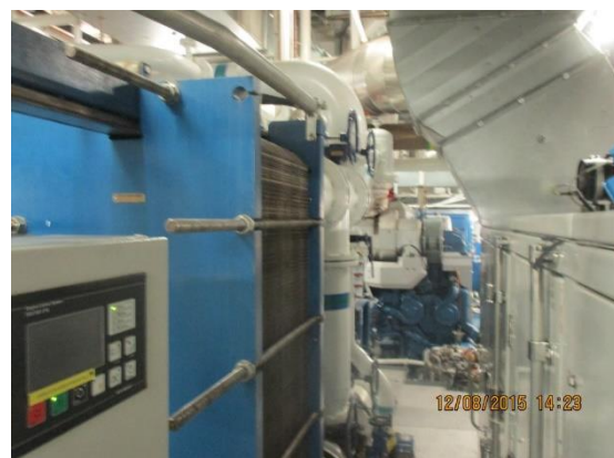
General view in the engine room showing one of the ME coolers
