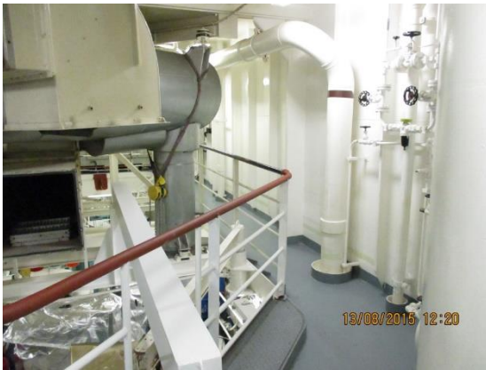
The Engine room was very clean and tidy
