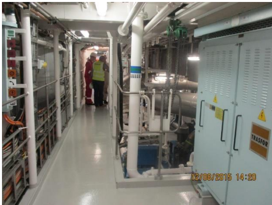
General engine room view showing the cleanliness
