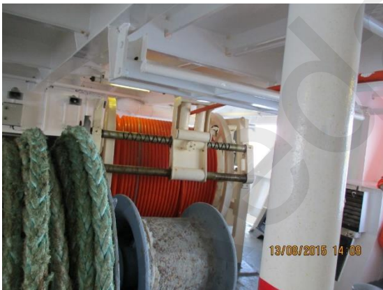
The flexible water pipe for servicing light houses
