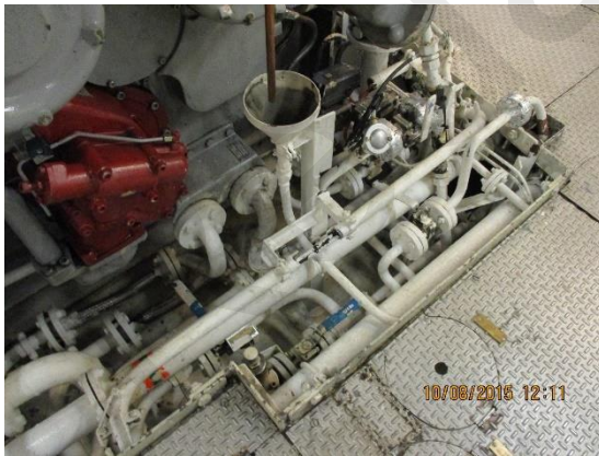
Engine room bilges are clean and free of oil/water.
