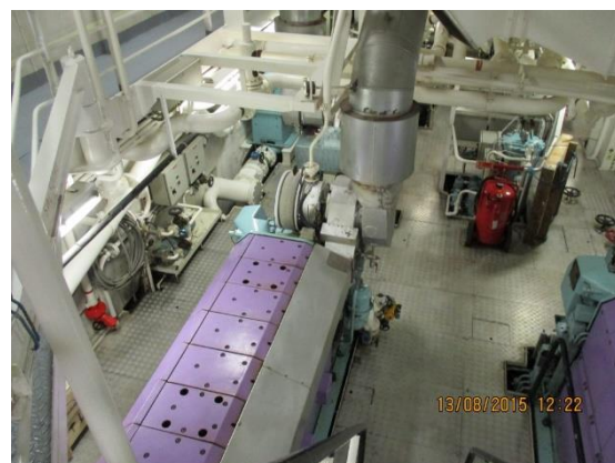
One of the 5 Main Generator Engines
