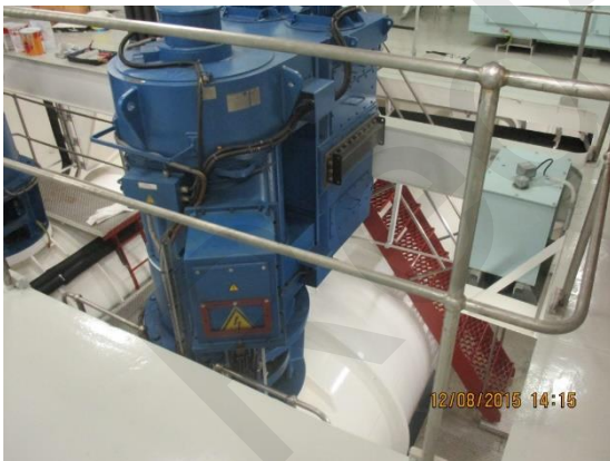
Forward machinery space showing one of the thruster motors
