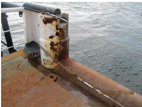
Area at the vessel's side where buoy work and chain maintenance is carried out. Only superficial damage to the paintwork was noticed.
