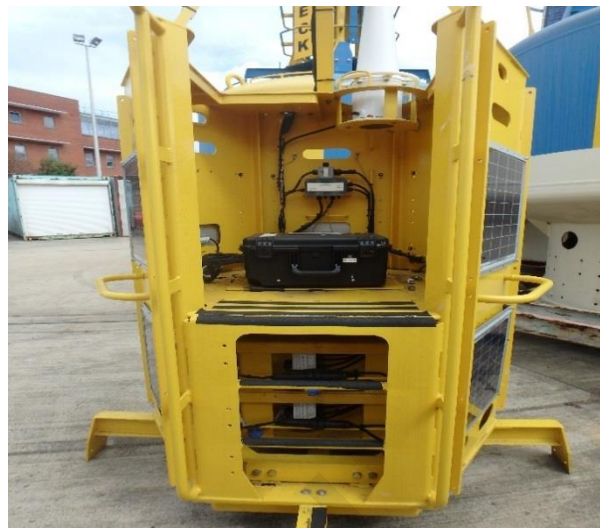
Photo 40 New electronics box inside the buoy top structure.
