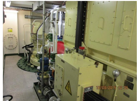
DP room aft showing one of the Rolls Royce Stern Azimuths (above)
