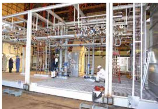
Air Handling Units for Concourse A at Heathrow's Terminal 5
