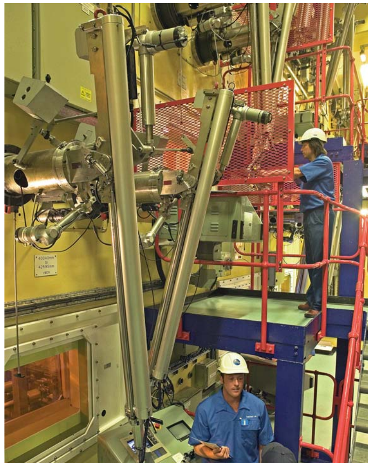
Above: One of the manufacturing lines where the highly active liquor is mixed with glass.
