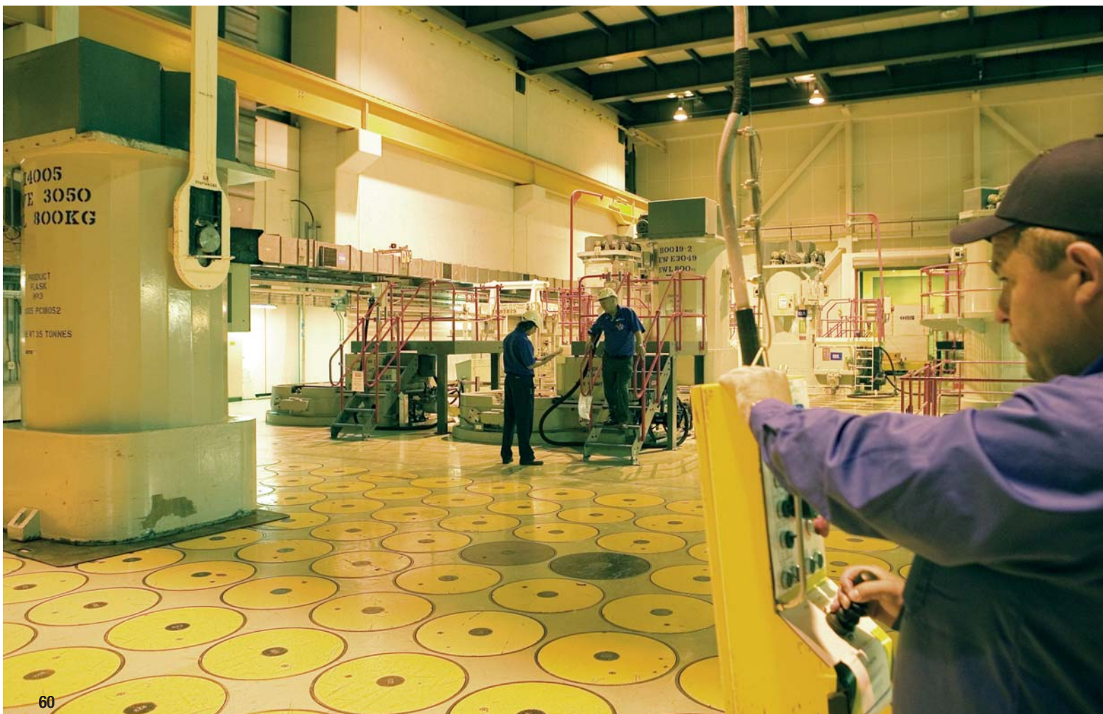
Below: The containers are kept in storage in the Vitrified Product Store.
