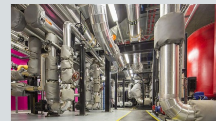
Kings Cross Energy Centre and CHP engines Source: www.kingscross.co.uk/
