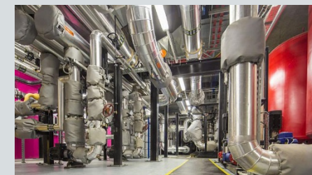
Source: www.kingscross.co.uk/ Kings Cross Energy Centre and CHP engines
