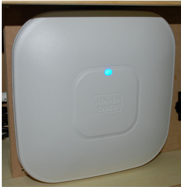
Figure 8 - Example of the Wireless Access Point (WAP)
