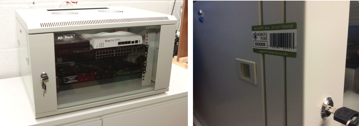
Figure 7 - Example of a cabinet housing the LAN Server, Network switch, LAN router and the security sticker placement
