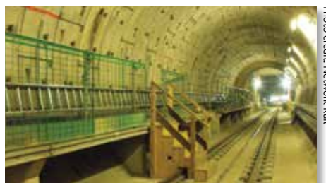
Canal tunnel This entirely new section of infrastructure will link the East Coast Main Line with the core Thameslink network and radically enhance the range of destinations connected to Cambridge. It could also connect to the proposed Science Park station.
