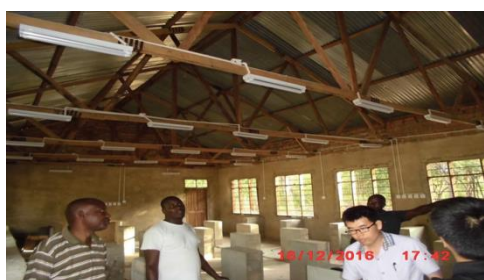
A school laboratory room with excessive light fittings
