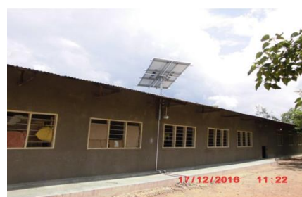
Conduits running direct on floor without being concealed or protected against mechanical damage.
