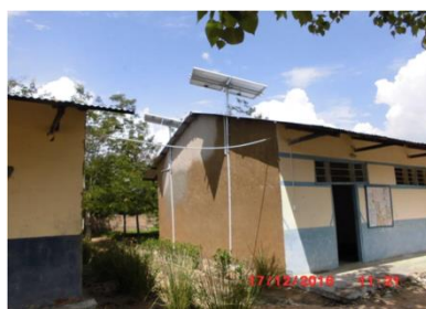
Conduits crossing from one building to another without a supporting wire.
