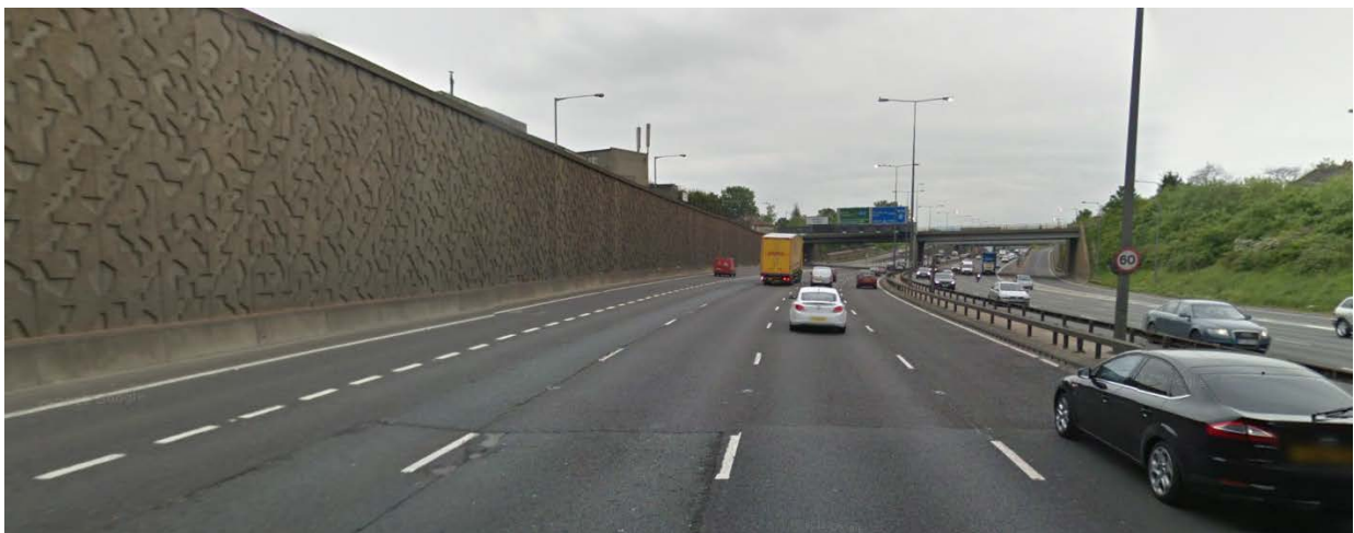
Image 2 – A282 southbound approaching Junction 1b showing retaining walls and adjacent private land
