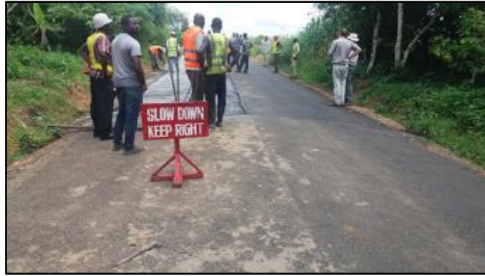
Figure 1: Inadequate Accommodation of Traffic for Obomfo-Densua Road Works
