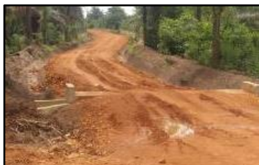
Poorly constructed Wingwalls
