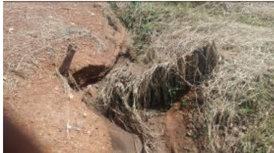
Poorly maintained scour checks
