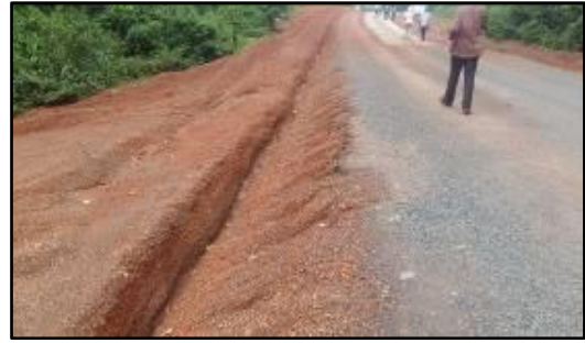
Erosion development in side ditch along steep slope of sealed low volume road
