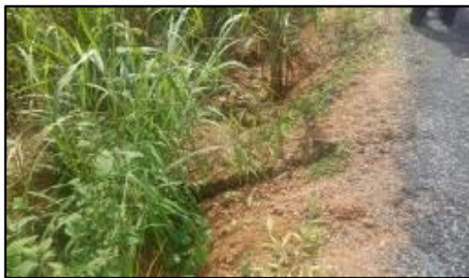
Poorly maintained scour check
