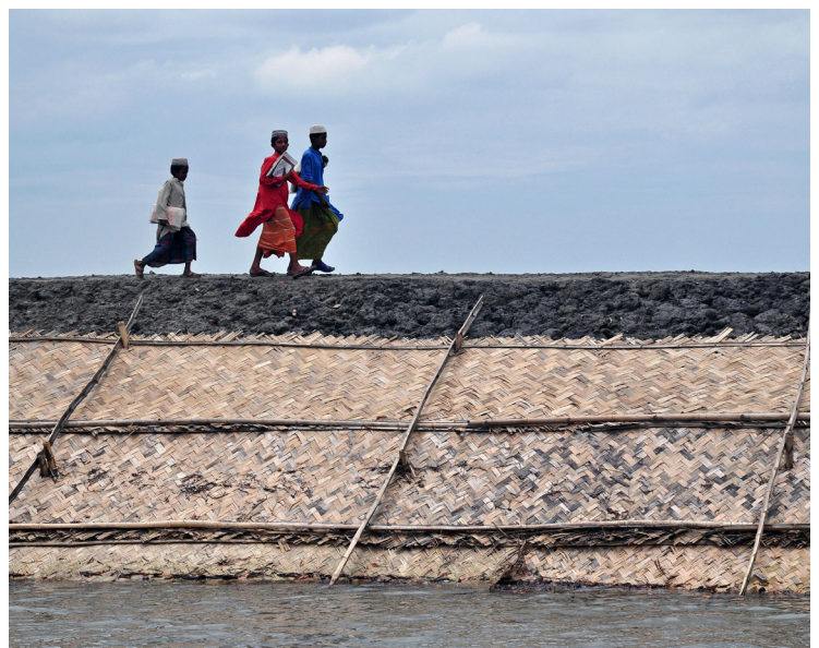
A remodelled embankment with a protective shield provided by the Government of Bangladesh in preparation for the monsoon season.
