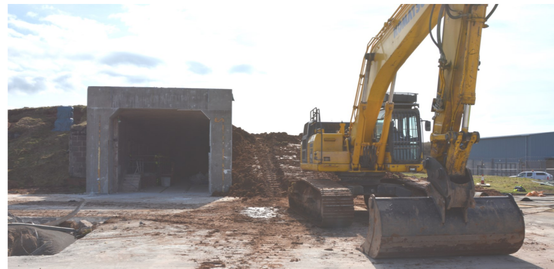
All change: above, the Retrieval Facility has gone and the entrance to Magazine 4 is visible., and below, as it previously looked with the old MRF in the foreground.
