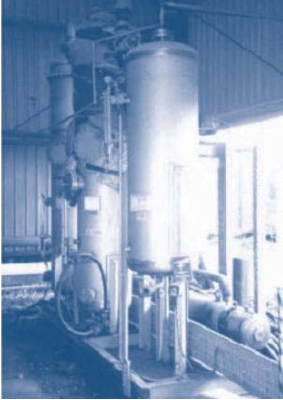
Figure 5.5 A UK pilot-scale scrubbing plant based on a hydrocarbon oil
