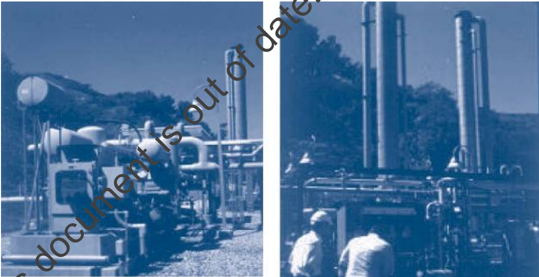
Figure 5.6 Selexol™ plants at Brea Olinda and Mountain Gate landfills in California
