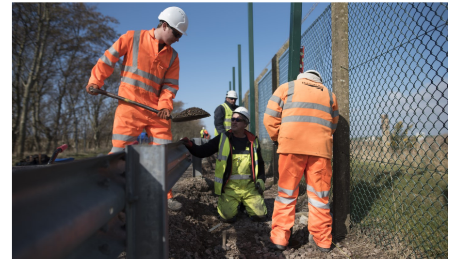
Digging it: Work on installing posts for the new fence last year, when sections of the old fence were still in place
