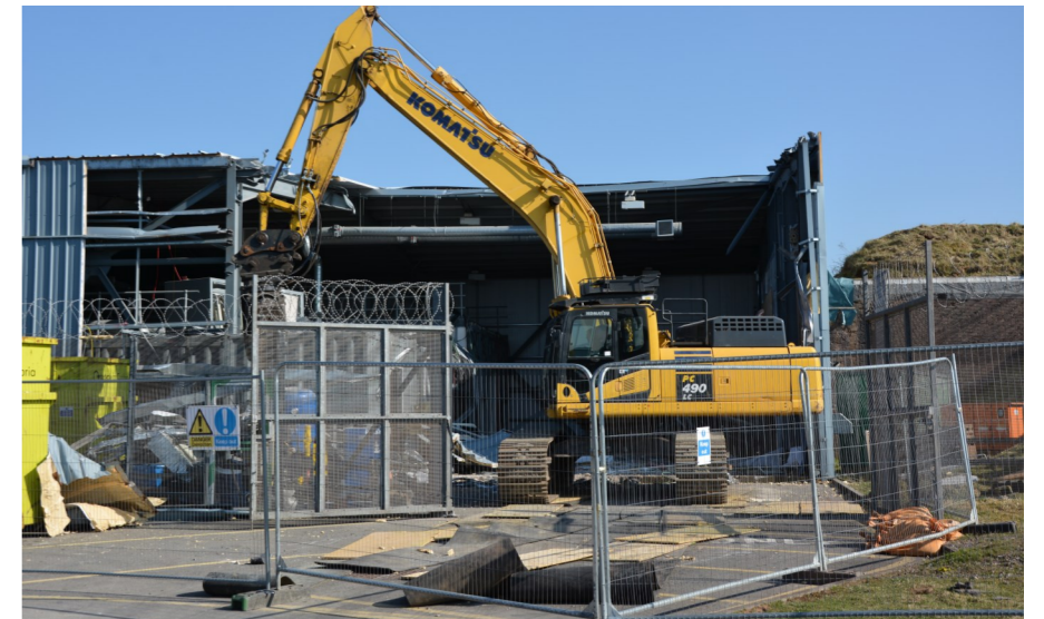
Skyline change: The demolition of Magazine 4's Retrieval Facility on our site was a major step forward for the PCM team
