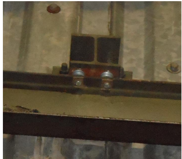
Photo 4 Adjacent bracket with washers in lieu of shim
