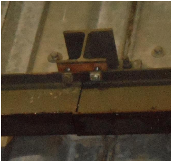
Photo 3 Bracket with shim missing
