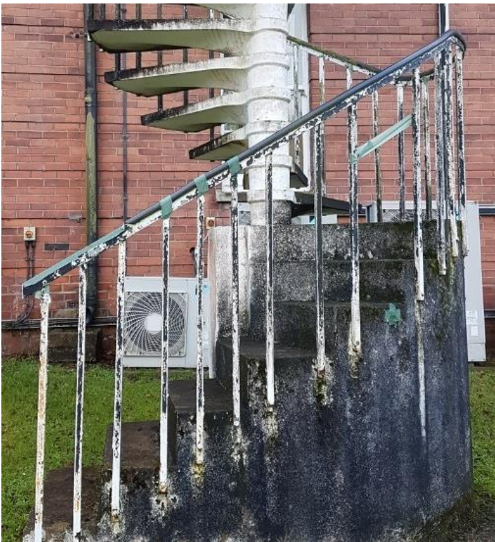
Photo1 Fire Escape showing PVC tape repairs
