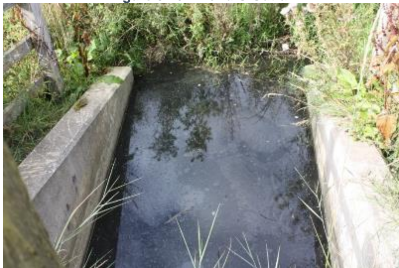
Figure 5.26 – Pond C Outfall
