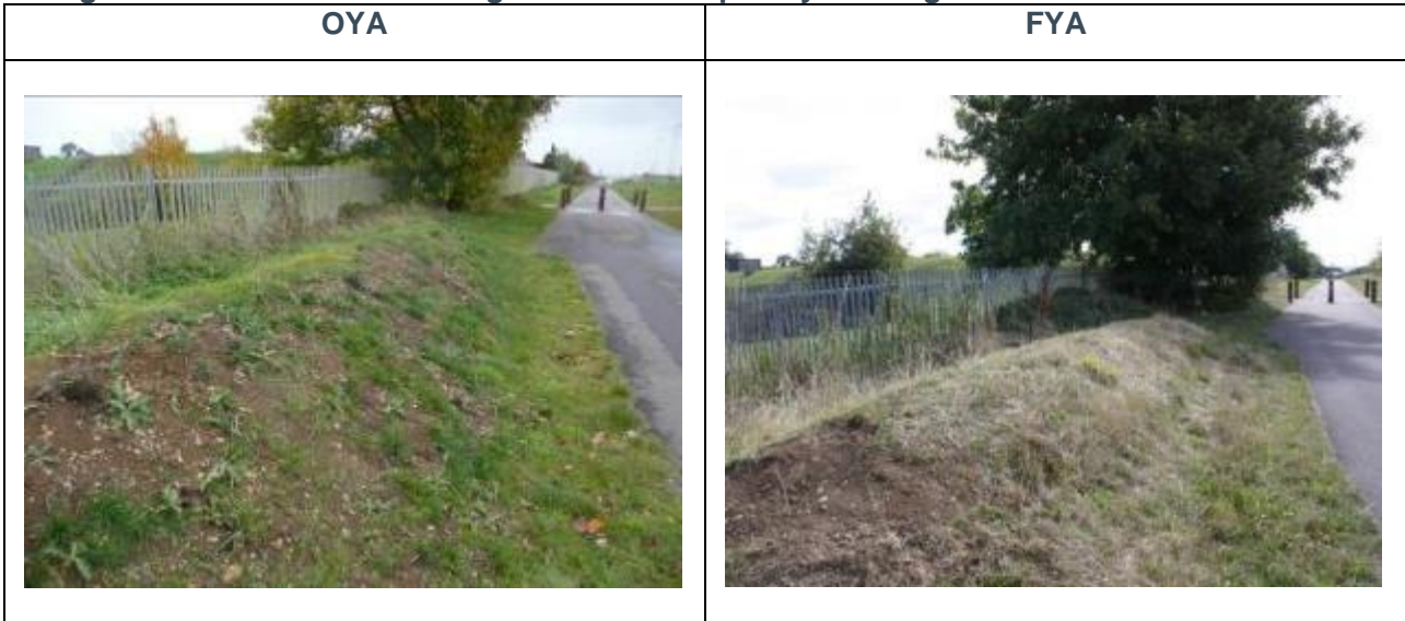
Figure 5.19 – Earthworks along old A419 with patchy seeding and weeds at OYA and FYA.
