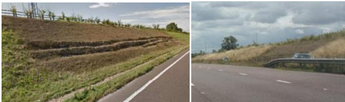
Figure 5.12 – Rocky outcrop left exposed on the northbound carriageway (image on the left taken from Google Maps, dated September 2012, image on the right taken during August 2014 site visit)
