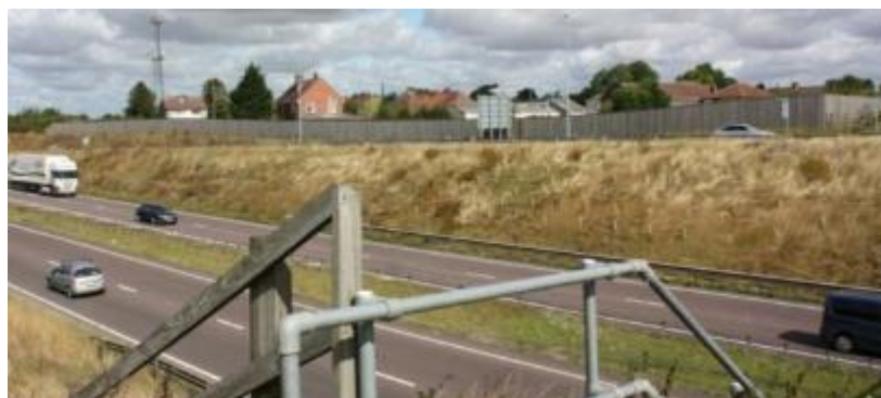
Figure 5.6 – Environmental barrier near Lady Lane Overbridge (view looking north across the bypass)
