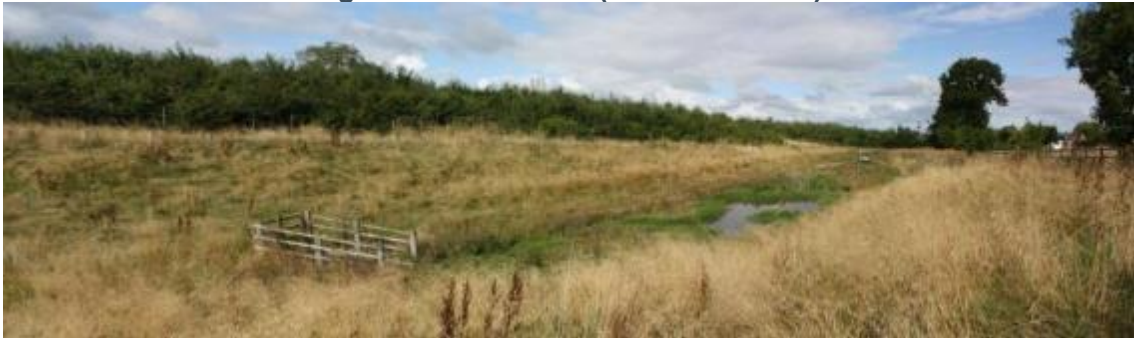
Figure 5.29 – Pond C – gate is unsecured and lifebuoy missing
