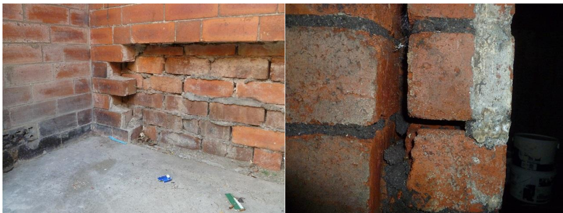
Figure 3-5 The difference in quality of brickwork between inner and outer leaf of a solid wall and the finger cavity between the them
