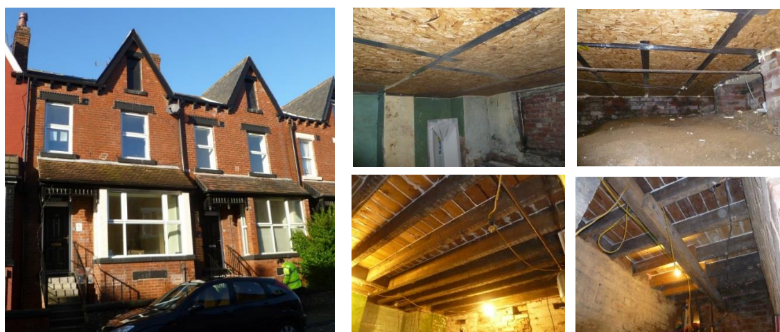
Figure 3-3 Dwellings I-02 & I-03, and the different treatment of the suspended timber ground floor, views from the cellar; top – contractor retrofit, bottom – local housing charity retrofit prior to insulation installation
