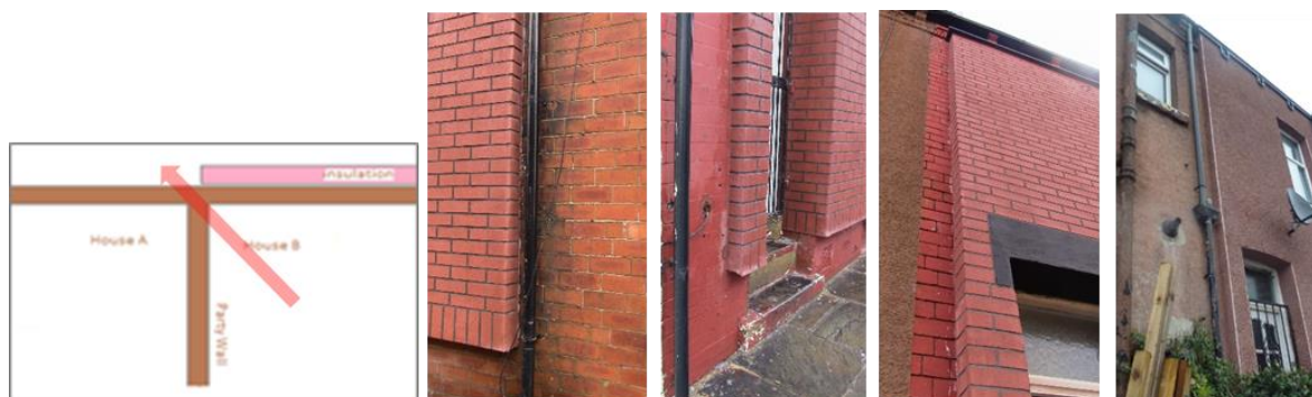
Figure 2-12 Thermal break at party wall/external wall junctions between differently owned terraced properties
