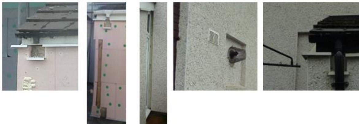
Figure 2-7 Thermal breaks at insulation cut-outs at external pipes, services, walls, doors etc: these are typical for 1945-1970s system built properties where these services are not being amended in the EWI works
