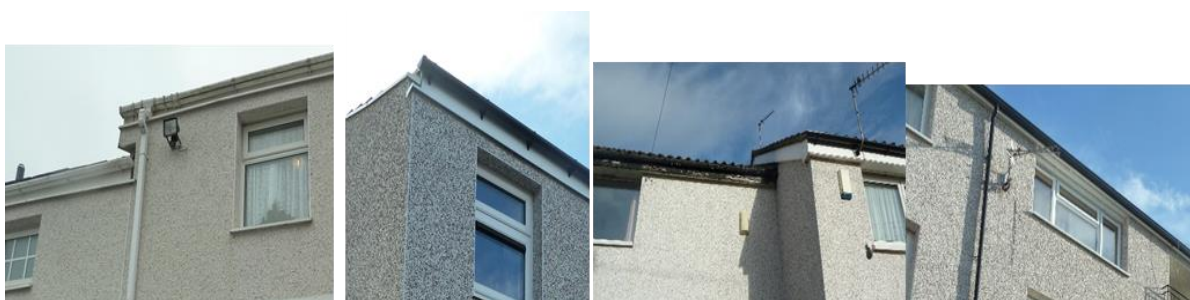
Figure 2-3 Thermal breaks introduced to top floor wall/ceiling junctions: 1945-1970s system built, including flats, terraces and semis. The roof, eaves and sometimes rainwater goods are not amended for the addition of EWI
