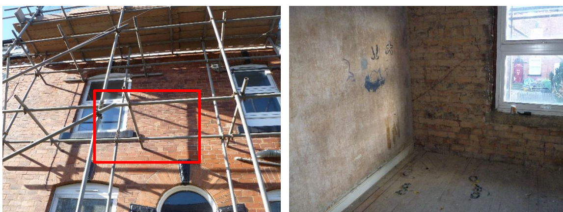
Figure 3-6 Dwelling C-02 prior to application of IWI insulated plasterboard on the external wall and plasterboard on the internal wall.
