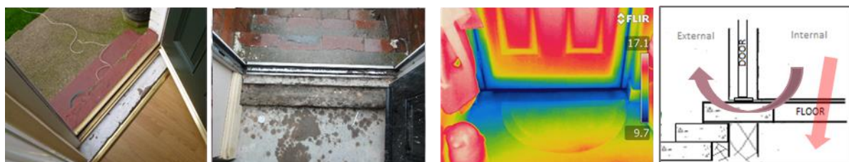
Figure 2-10 Thermal breaks due to lack of insulation to ground floor and single slab door thresholds. These thresholds are found at suspended timber or solid concrete ground level floors
