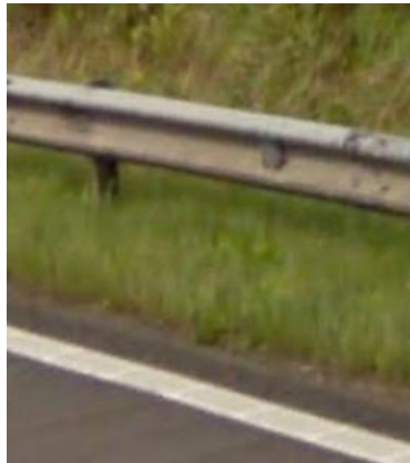
Figure A11.1 – Barrier Reflectors
