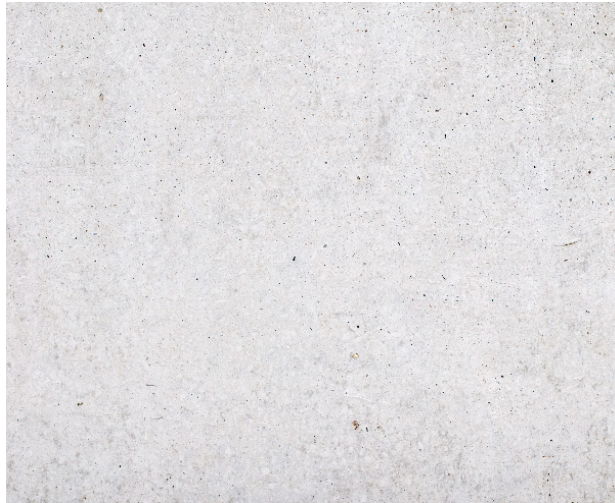
Good concrete colour and finish must be an aspiration in the construction of this bridge. The use of granulated blast furnace slag along with the cement can help to achieve a light colour, minimising the embodied carbon
