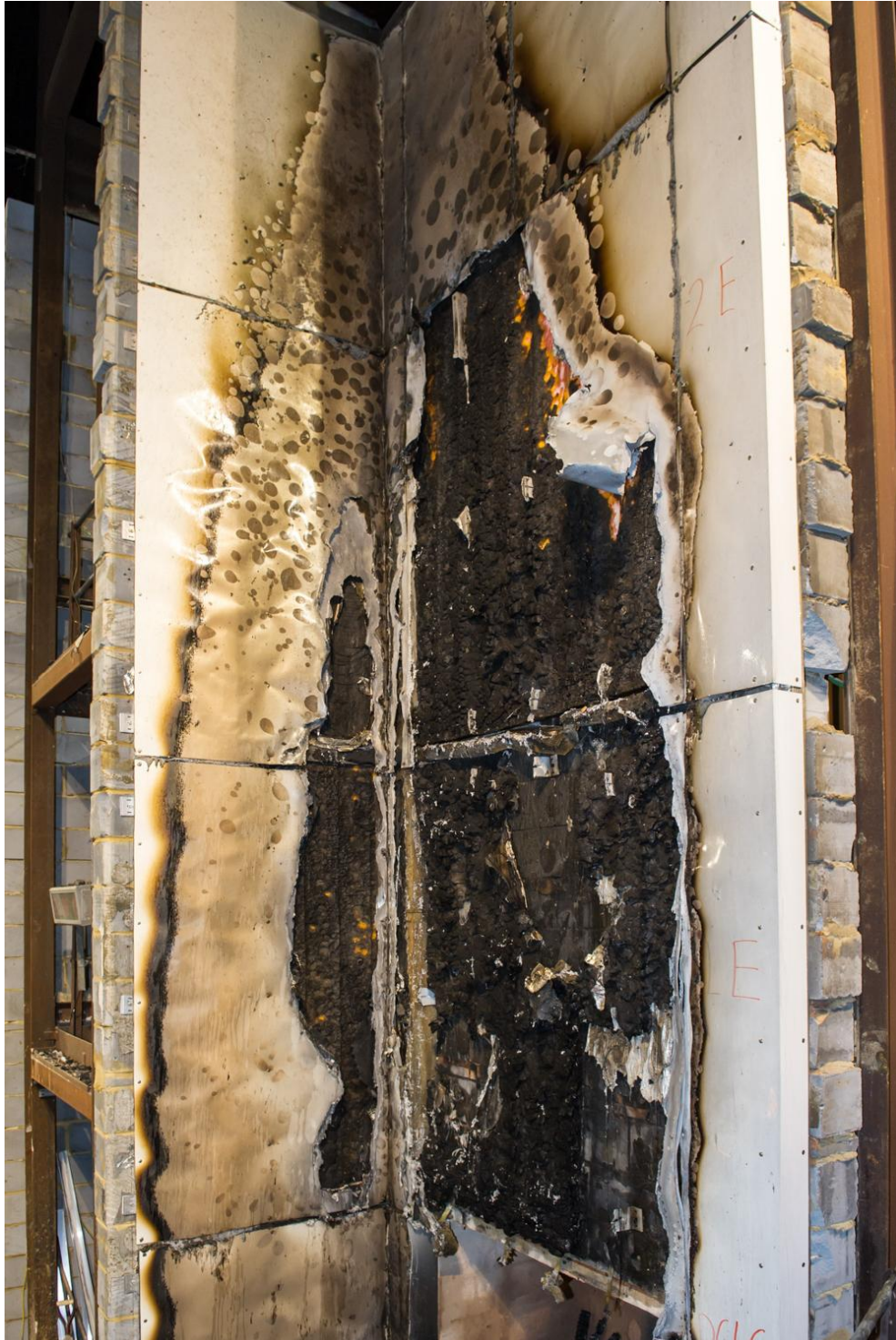
Figure 23. Photograph of system post-test – wing wall.
