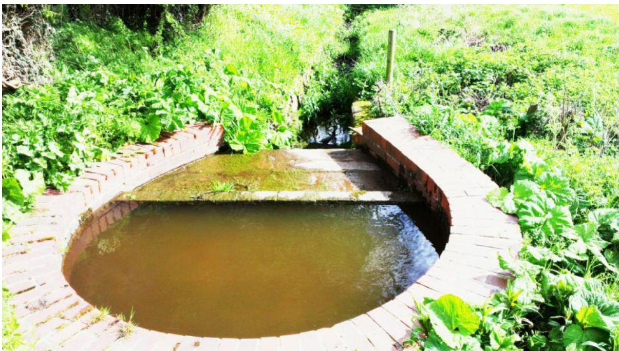
Location P17 – Example of Pipe and Weir overflow to control levels in the canal, flowing toward the River Trent.
