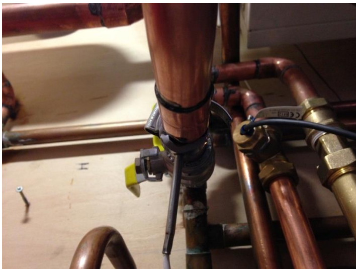
Figure 5-9. CS12 - Close up of pipework showing insulation between temperature sensor and pipe (centre of image). The external temperature sensor for the heat meter can also be seen, just right of centre, in a pocket
