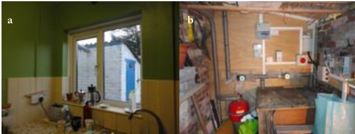
Figure 5-18. CS20 - (a) View from the kitchen to out-house and (b) installation of buffer vessels and pipework in out-house
