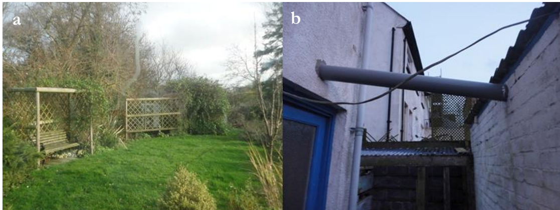
Figure 4-8. (a) Outdoor unit behind trellis (CS09), (b) Insulated external pipework (CS20)
