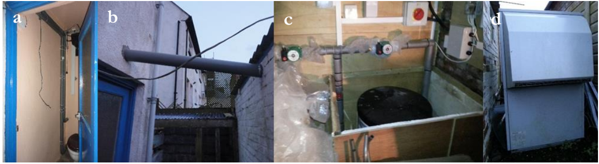
Figure 4-12. (a) pipes running through the externally accessed, unheated outdoor toilet, (b) between the house and the external shed, (c) circulating pumps, buffer vessel and heat meters within the shed, (d) external HP unit, located next to the shed (CS20)
