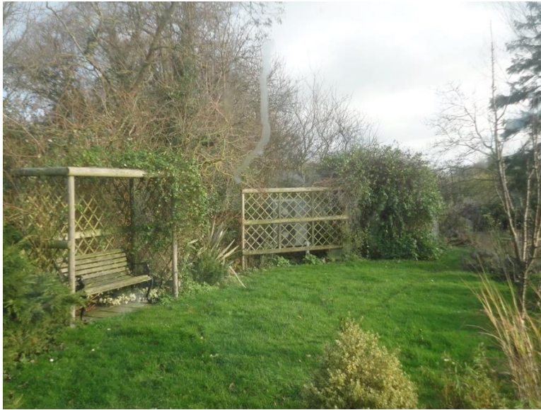
Figure 5-1. CS09 – External unit behind trellis in corner of garden
