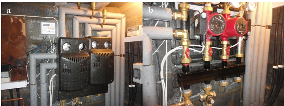
Figure 4-3. (a) High quality insulation of pipework in outdoor, unheated shed with and (b) with insulated pump and manifold covers removed (CS13)
