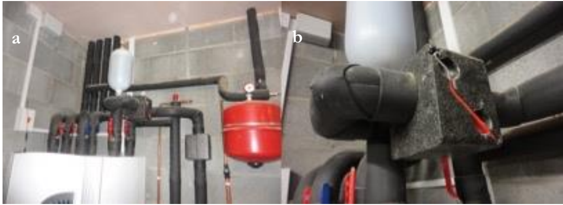
Figure 4-2. (a) Example of high quality insulation (CS15) and (b) detail of high quality valve insulation (CS15)
