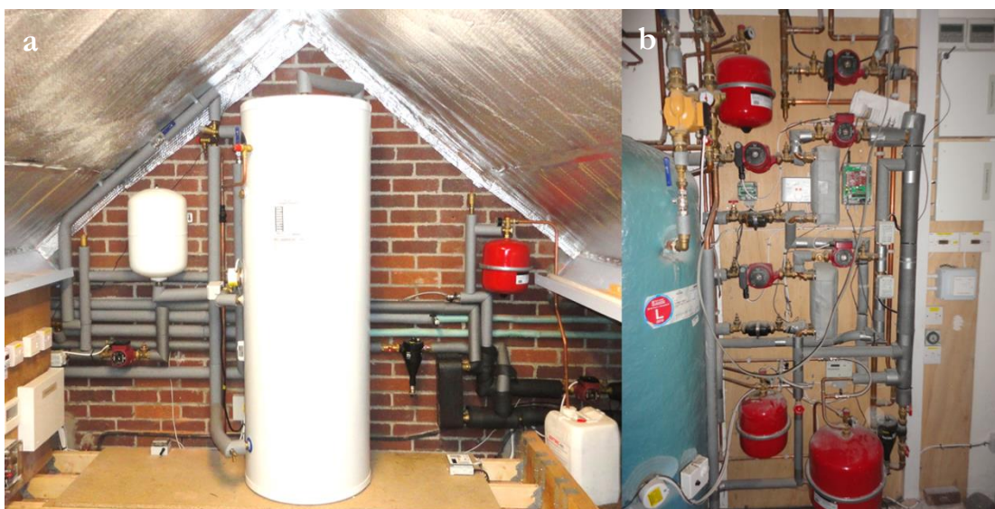
Figure 4-9. (a) Neat installation with plate heat exchanger (CS11), (b) Plate heat exchangers by the same installer (CS10)
