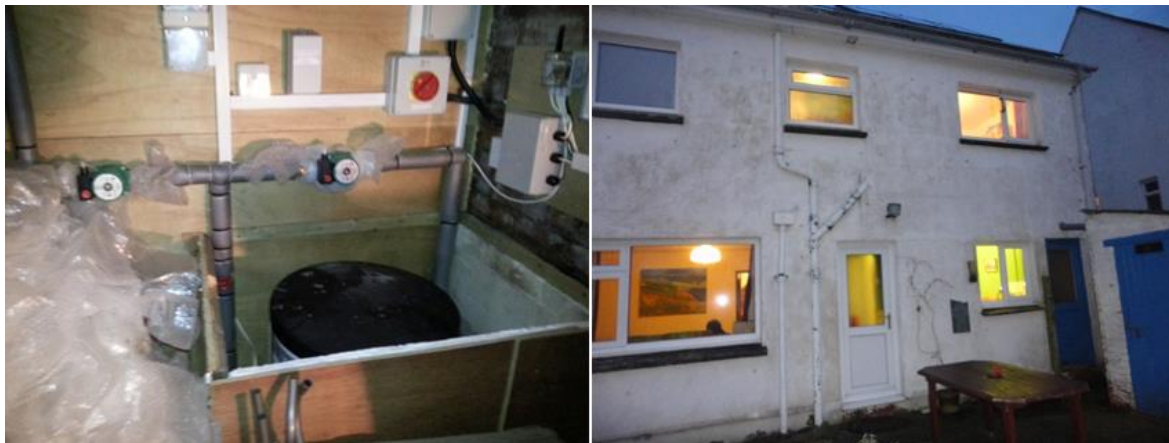
Figure 5-19. CS20 - (a) Buffer tank (with additional bubblewrap to act as insulation) and circulation pumps in unheated shed and (b) location of the shed, to the right of blue door
