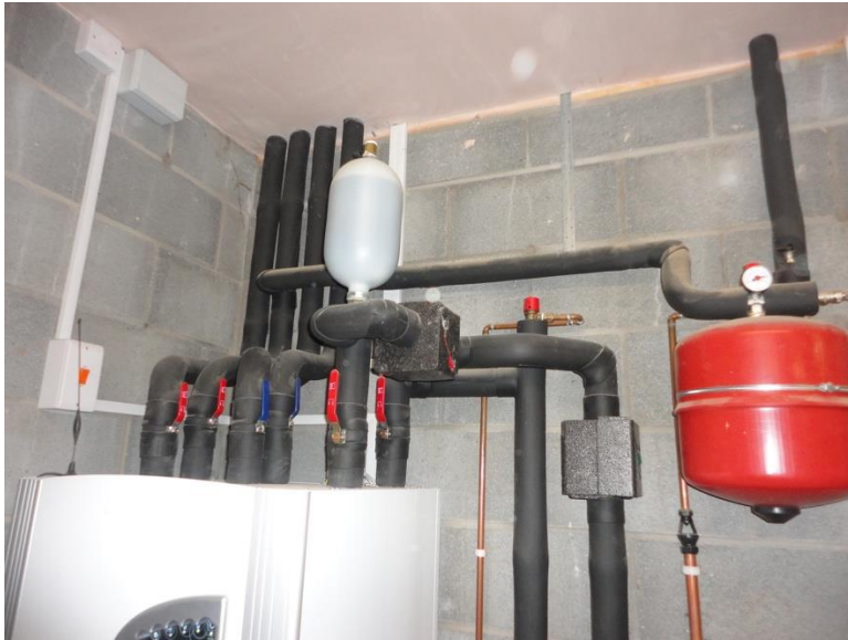
Figure 5-5. CS15 – High quality insulation and layout of pipework
