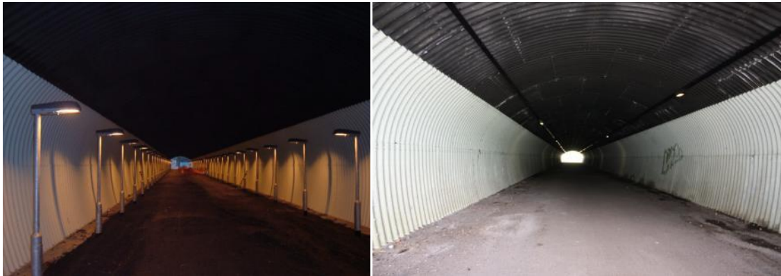
Figure C.2 – Nickey Line Underpass showing original lighting and new lighting installed in late 2013 along tracks on the upper part of the tunnel light.
