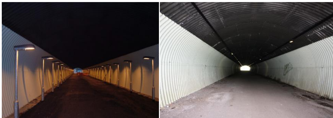
Figure 5.13 – Nickey Line Underpass showing original lighting and new lighting installed in late 2013 along tracks on the upper part of the tunnel light.
