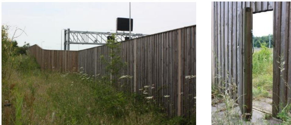
Figure 5.2 – Environmental Barrier adjacent to Slip End playing fields, including vandalised gate
