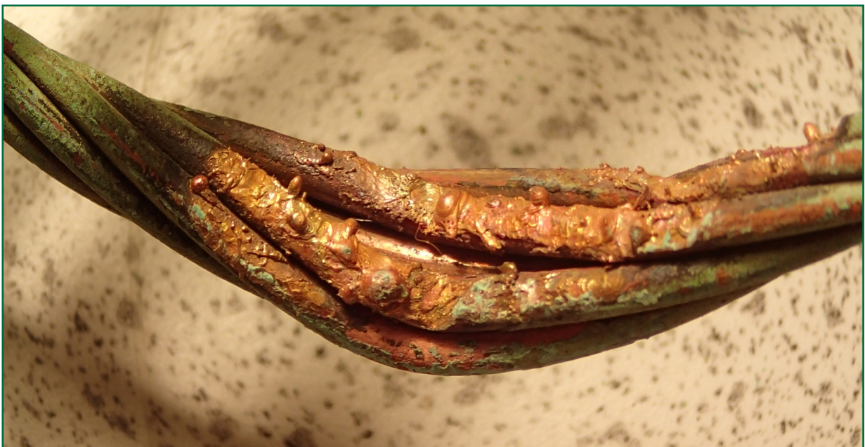
Figure 6: Electrical arcing damage on the London section of the broken auxiliary wire
