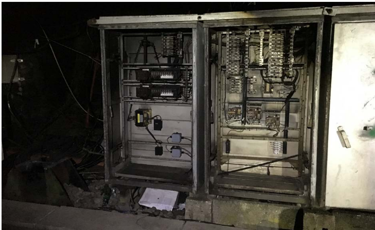
The location cabinets with missing doors (image courtesy of Network Rail)
