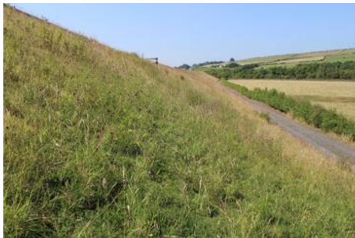
Figure 5.24 Example of species diversity establishing on embankment slopes at western end of the bypass on approach to river bridge
