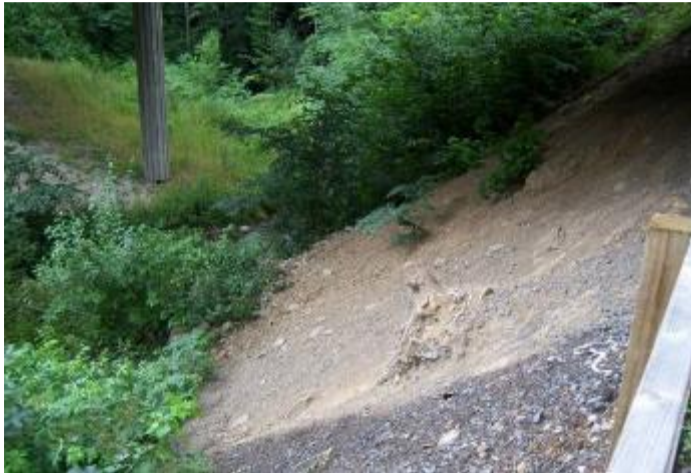
Figure 9.19 OYA Bare ground with potential to erode beneath bridge in Gees Wood
