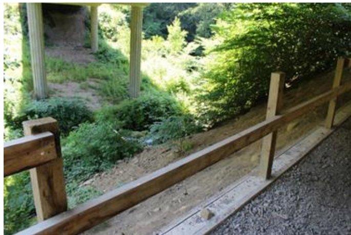
Figure 5.23 Vandalised post and rail fence within Gees Wood
