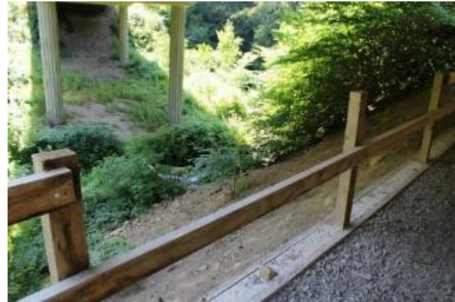
Figure 9.20 At FYA, there remains limited grass / scrub growth due to the dry and shady conditions beneath the bridge. Vandalised top rail can be seen used as a plank to cross Langley Burn.
